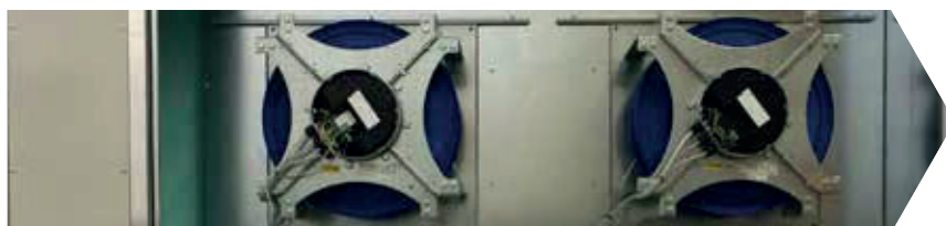
Modulating fans and high efficiency filters
